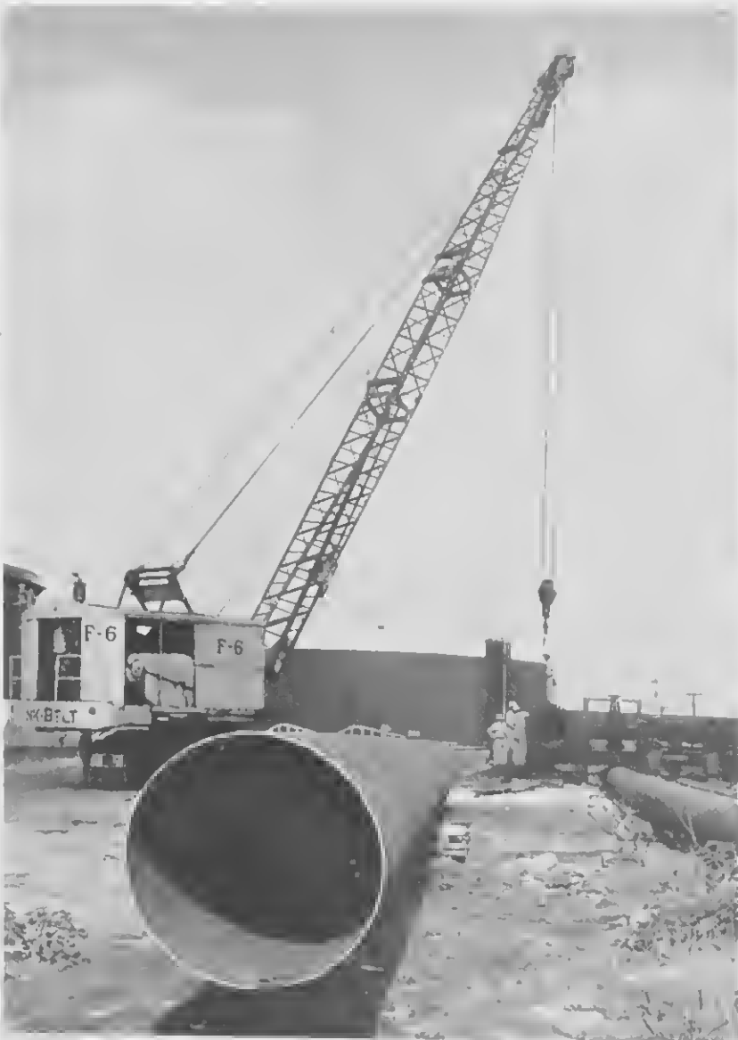
FROM THIS angle the 36-inch pipe looks even bigger. It will be able to handle 30,000 barrels an hour.
